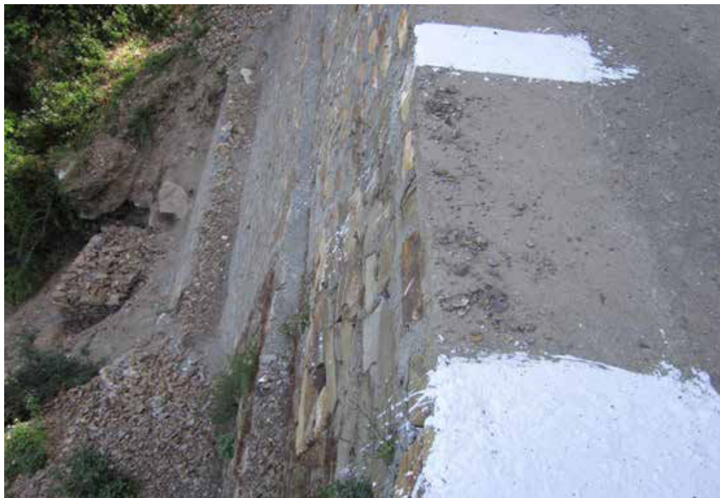
Picture 6 Wire-Crete & Retaining wall constructed along the chainage 1 + 950 Km on Chailusain-Devikhet road.
